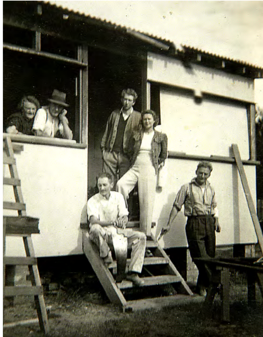
Building the house on the property adjoining the lake. When Uncle Jack died in his nineties it was worth over a million bucks.
